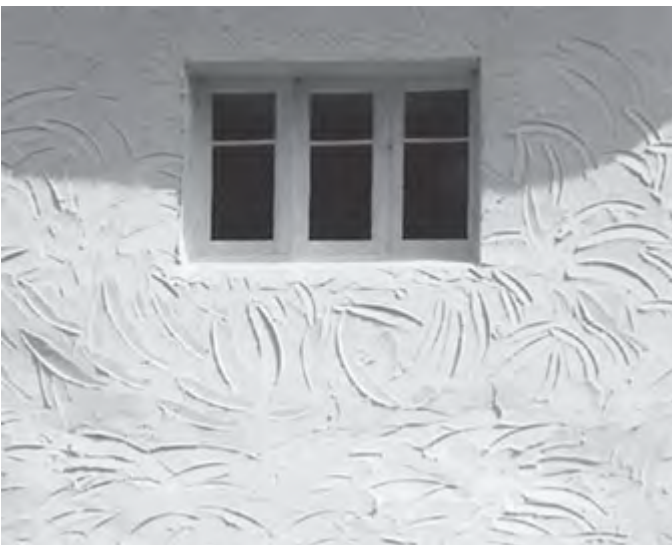
Figure 53 Renewing the render of this cottage was appropriate, but not the added patterning
