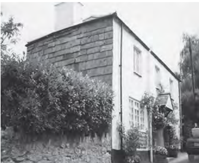
Figure 51 This prominent slate cladding is attractive, but its use can be rare and needs to remain so to preserve its particular identity
